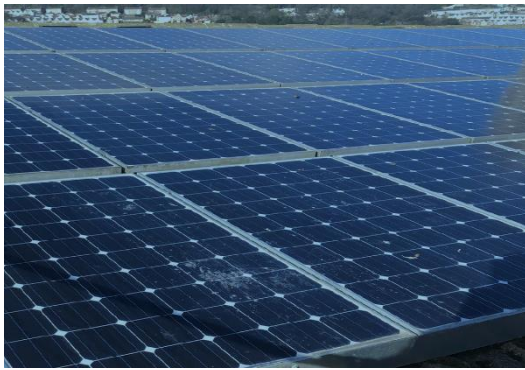
Solar PV modules installed on the Guildhall
